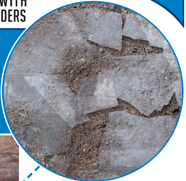
6 mil Polyethylene Vapor Retarder Failure
